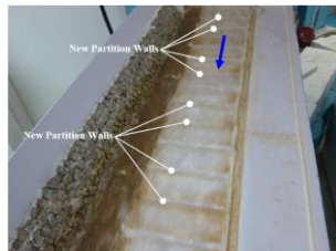
Partition of additional boulder trap
